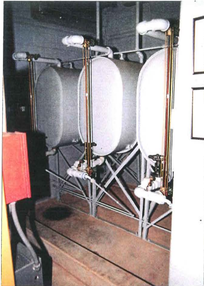
Photo 6-7. Fuel oil tanks for diesel engines in pumping station
